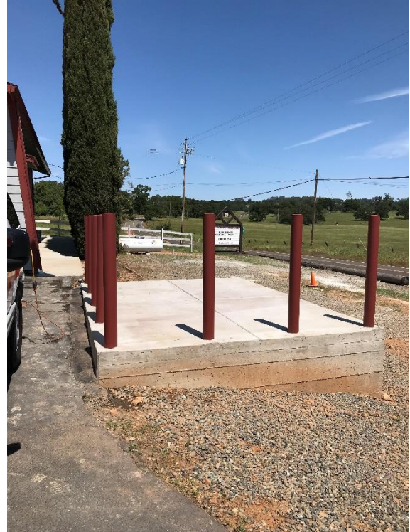
Fuel Cell Pad – Southside of Station
