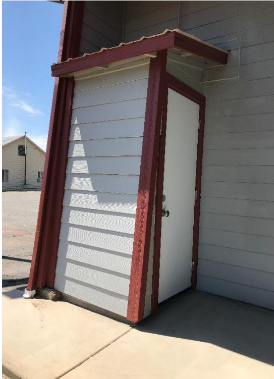
Air Compressor Room – Southside of Station
