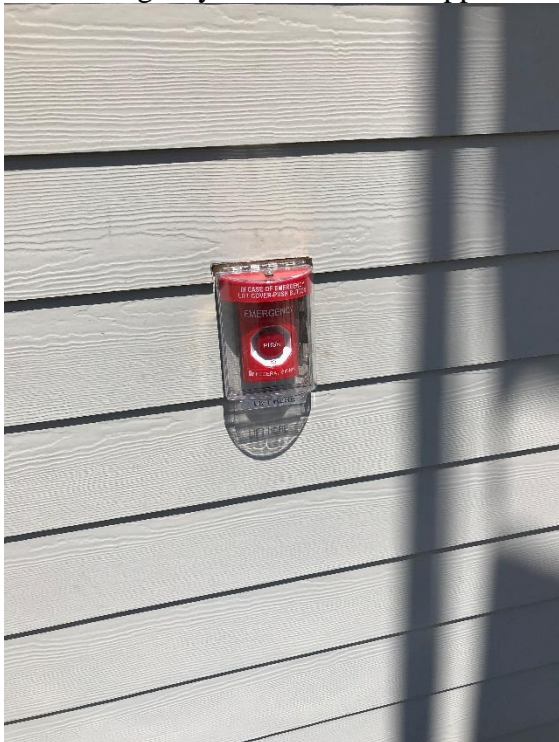
Fuel Emergency Shutoff – Near Apparatus Bay
